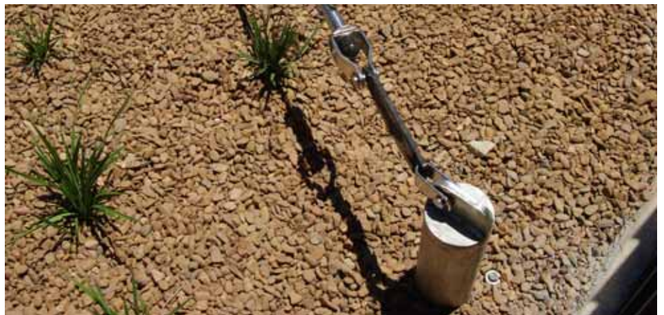
Cable anchor point on green roof at Adelaide Zoo (Photo sourced from Fifth Creek Studio)
